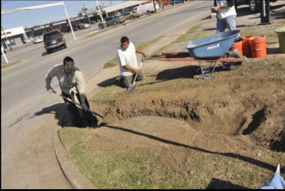
Work begins, digging a trench to lay out aggregate and collect water
